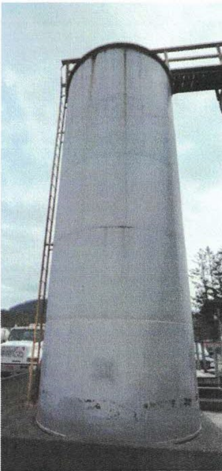
Figure 6 - Aboveground Storage Tank from CX 07
