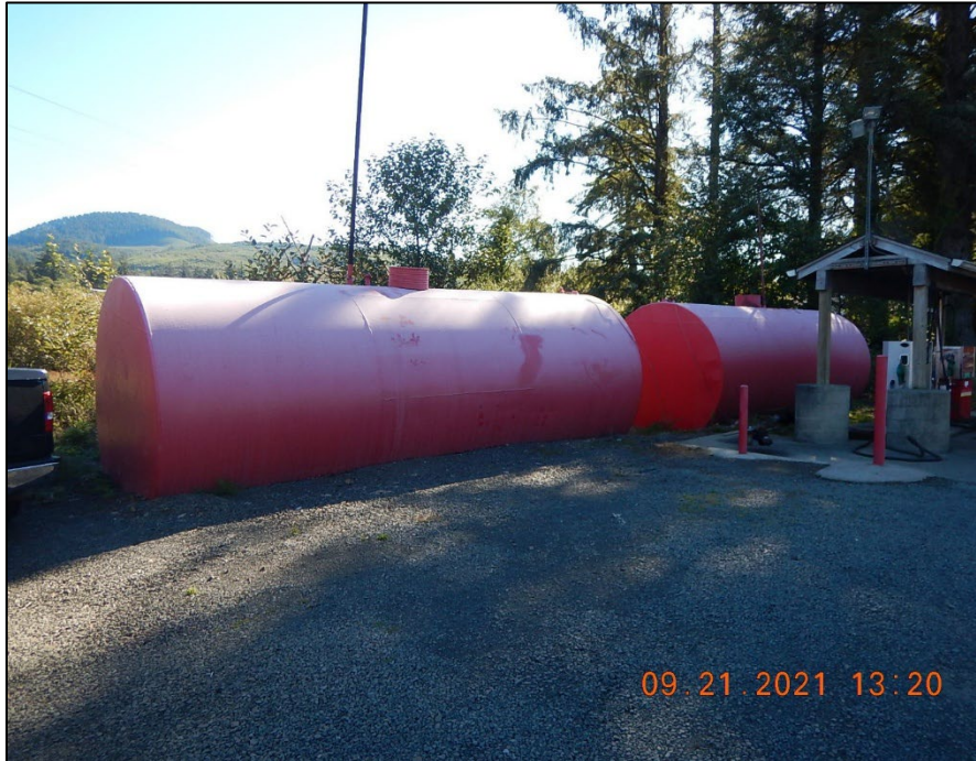
Figure 1 - Photo of Two 10,000-Gallon Aboveground Storage Tanks
